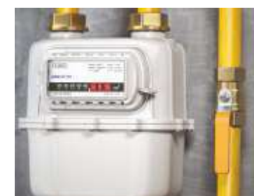
Piped Gas Facility
